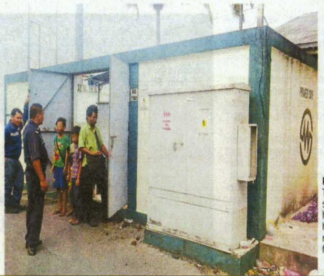
Risky stay The power sub-station has been home to a man and four boys.
